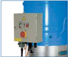
Control cabinet for motor, shaker and level sensor, as well as remote triggering via machine contact
