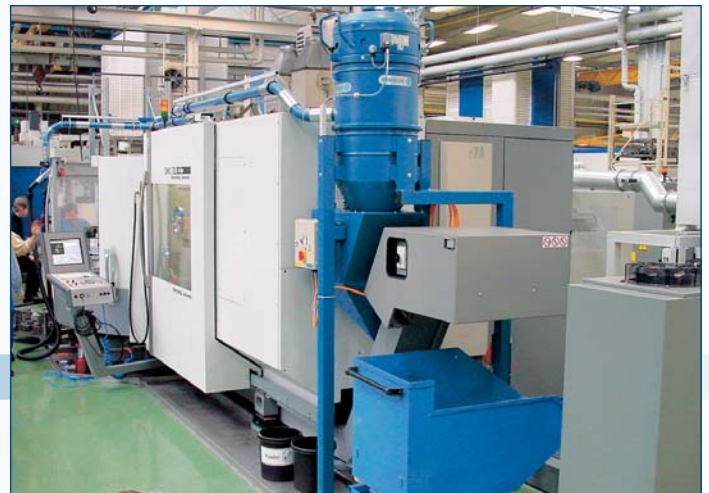
RI 750 with piping and suction point
