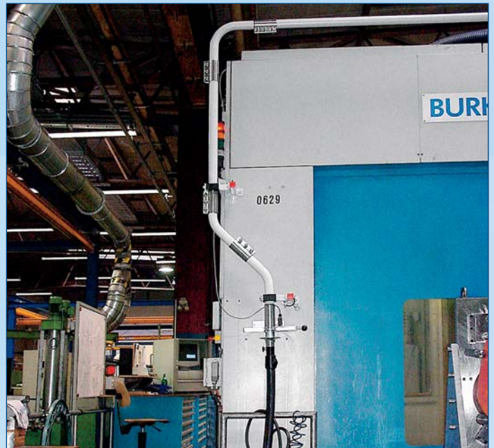
Picture on left: RI 751 with Ringler piping system and 2 suction points Picture on right: Suction point 2. The device switches off automatically when the suction hose is disconnected. The chips + coolant are automatically discharged into the chip conveyor on completion of the cleaning work.
